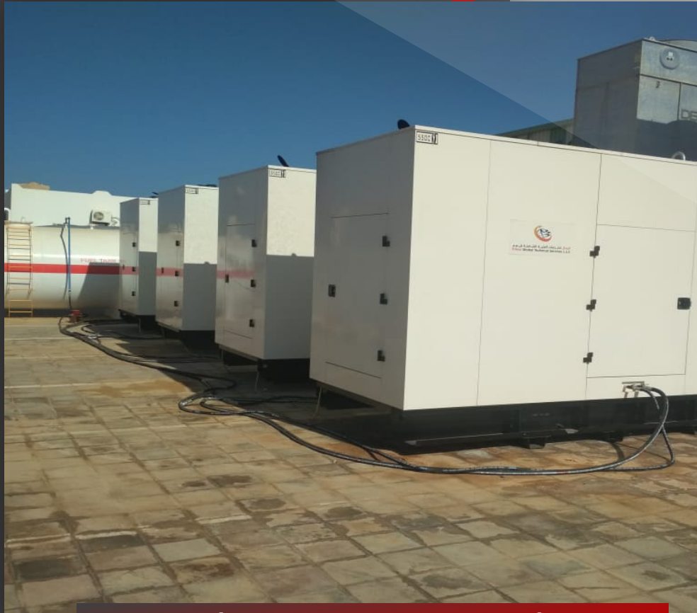
Special Economic Zone Authority Duqm - Generators (550 kVA) 2018
