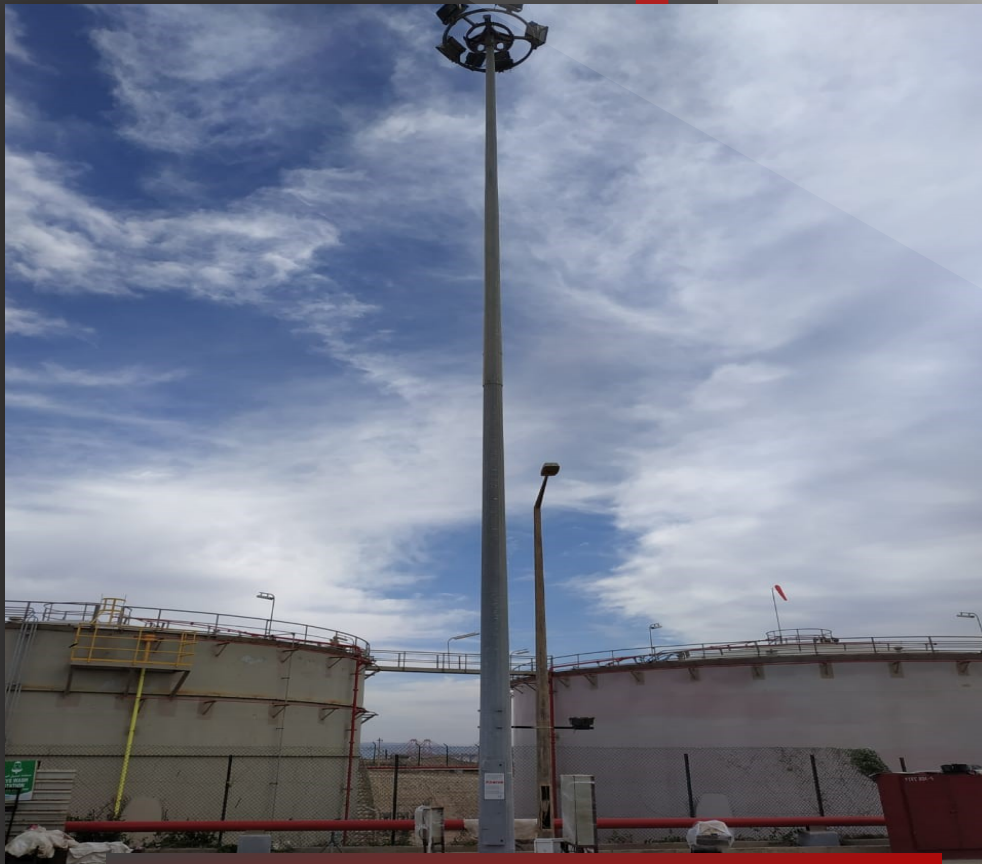
HIGH MAST LIGHTS – ORPIC RAYSUT TERMINAL PROJECT 2018
