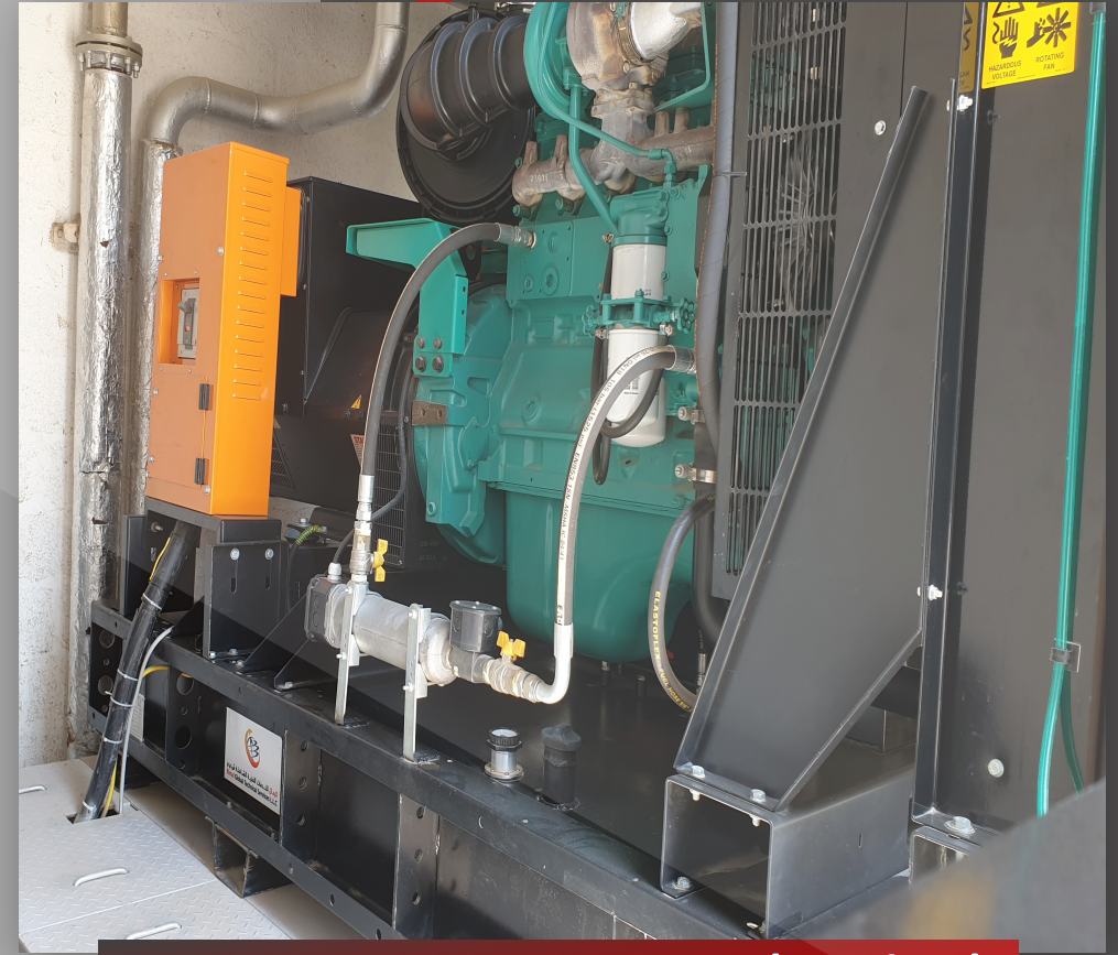
SQU DIESEL GENERATORS (275 kva) 2018
