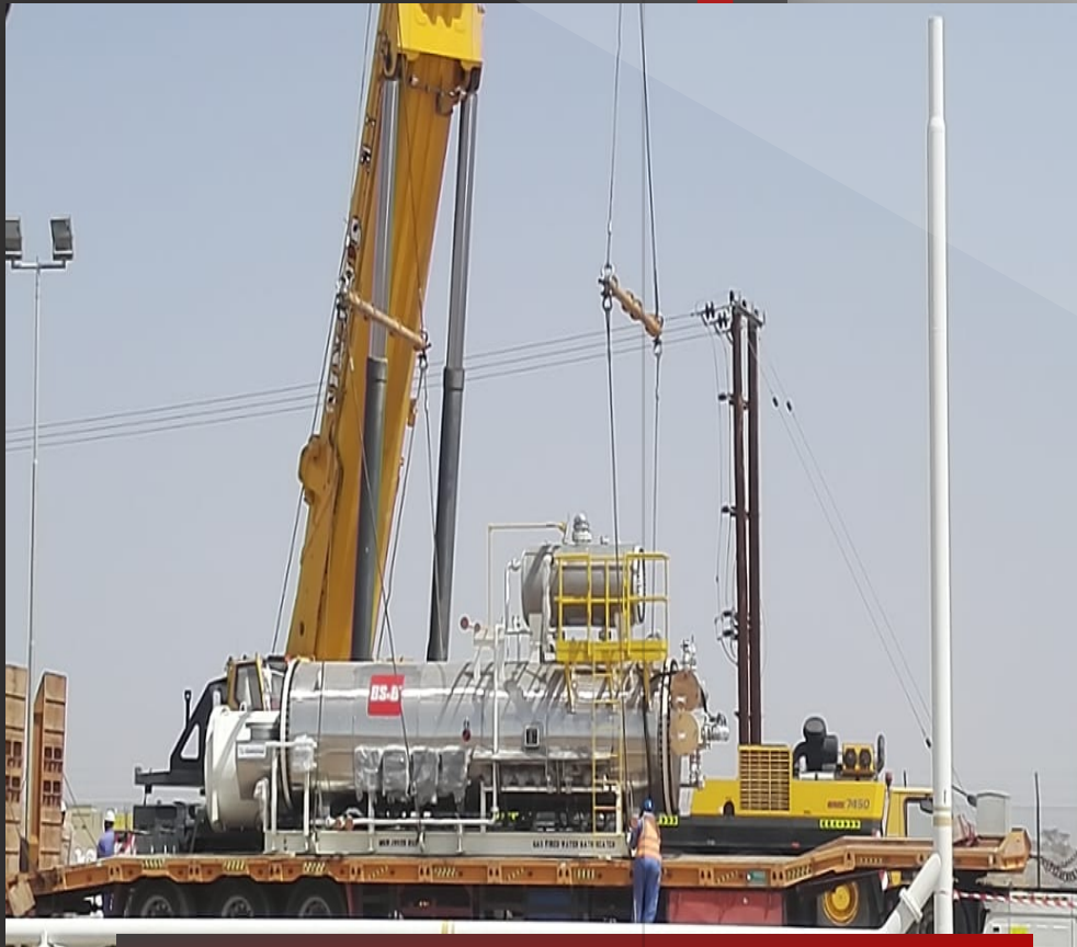
WATER BATH HEATER – SOHAR INDUSTRIAL ESTATE – OMAN GAS – 2019
