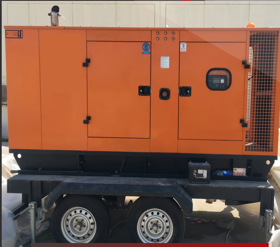
SSDC MOBILE DIESEL GENERATORS (220 kva) 2017
