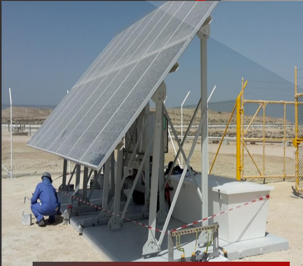
PDO OFF-GRID SOLAR SYSTEM – IN MARMUL 2019
