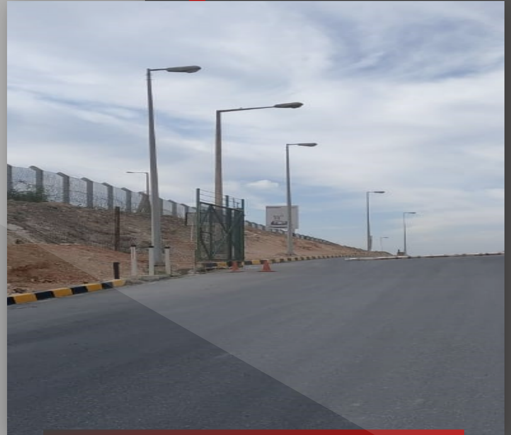
STREET LIGHTING – ORPIC RAYSUT TERMINAL PROJECT 2018
