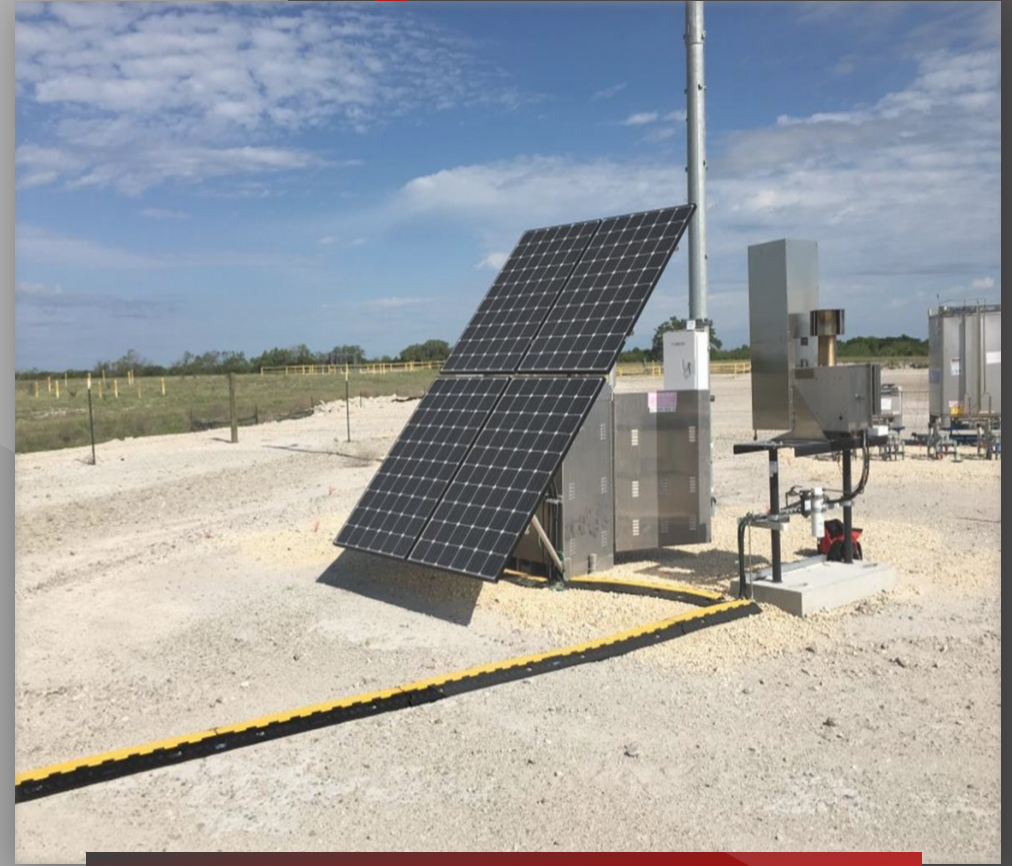
PDO OFF-GRID SOLAR SYSTEM - IN LEKWAIR 2019
