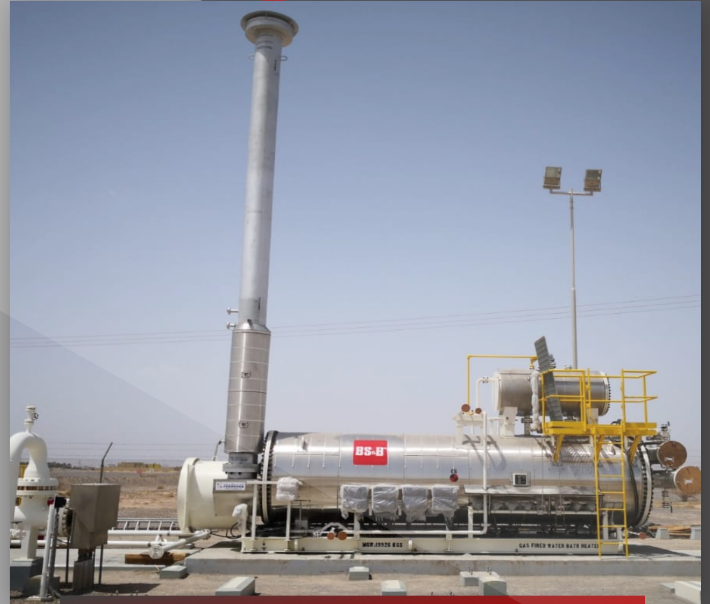
WATER BATH HEATER – MANAH INDUSTRIAL ESTATE – OMAN GAS – 2018
