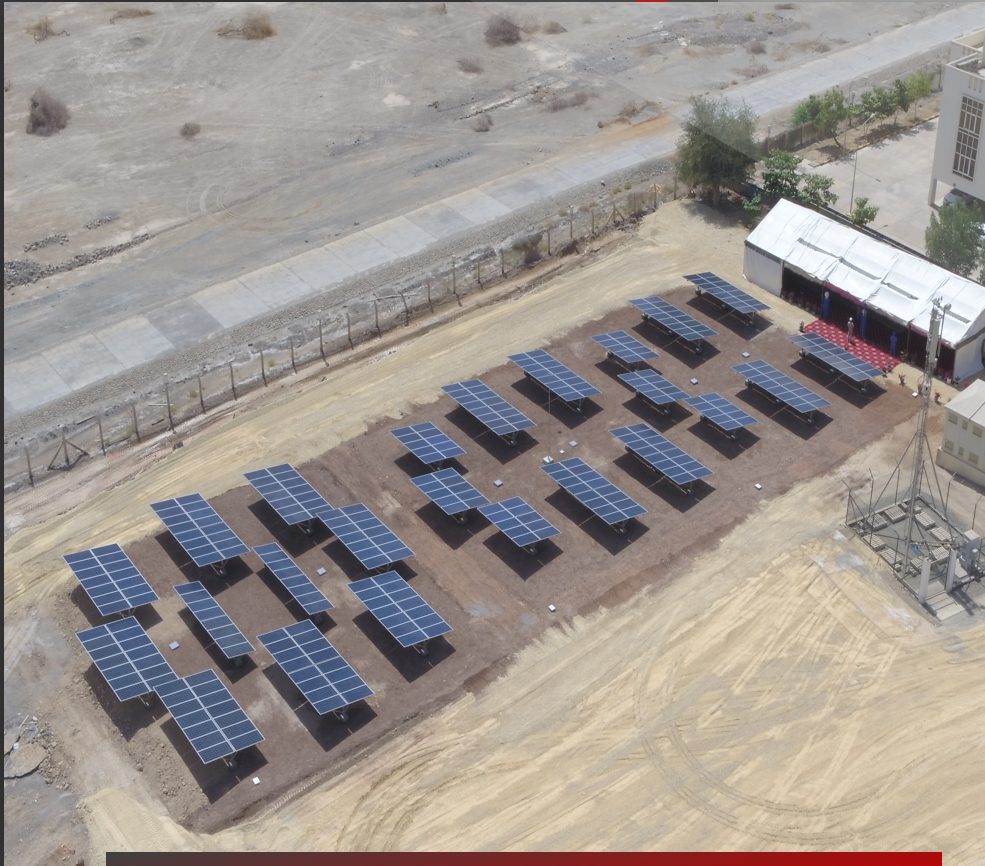
OMAN CEMENTS SOLAR POWER SYSTEM (100 KW) 2019
